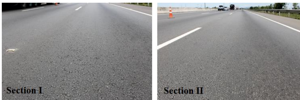
16 FIGURE 5 Appearance of the coating layer after three years of monitoring
