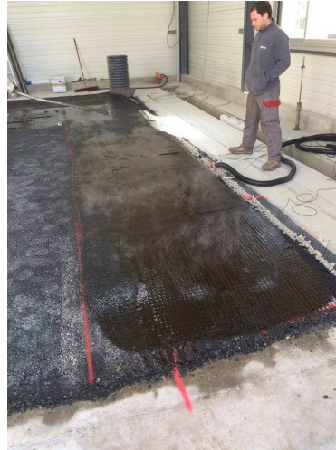
9 10 FIGURE 1 The second geosynthetic right after placement using the usual method for 11 reinforcement geosynthetics: the product is laid in the fresh tack coat emulsion.
