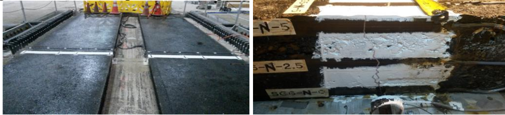
6 (a) Overlay Pavement (b) Crack through Strain Gage
